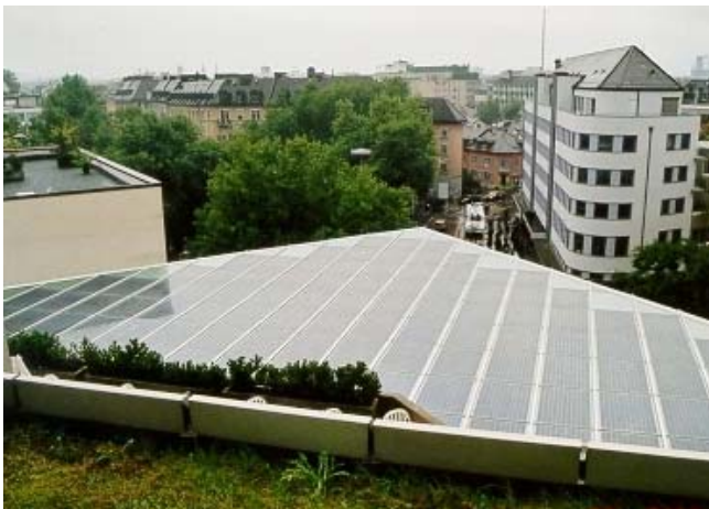
Custom-design, integrated glazed roof system, 30kWp, Switzerland
