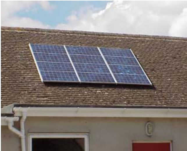
Retrofit standard system, 0.9kWp, UK
