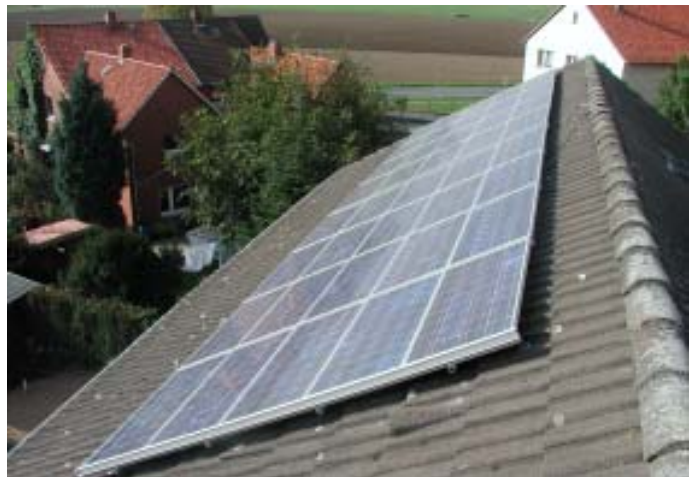
Solar modules can easily be retrofitted over existing roof in a cost-effective way.
